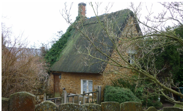
Above: 4 Church Lane, Hornton (before repair)
