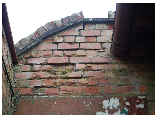
The buildings at RAF Bicester remain in poor condition whilst the Crichel Down process is concluding
